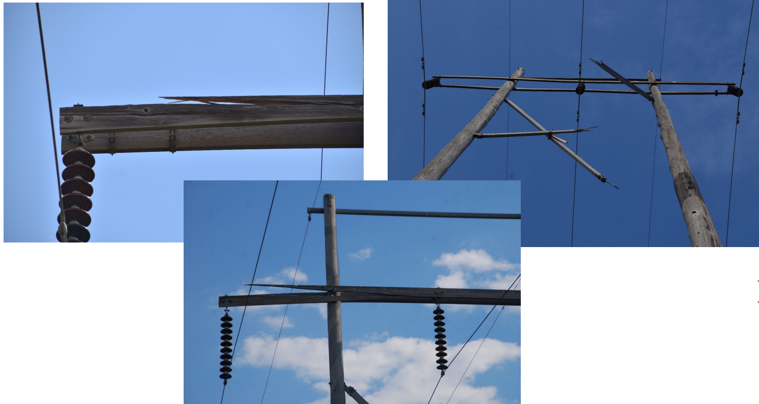
Broken, Split Cross Arms
