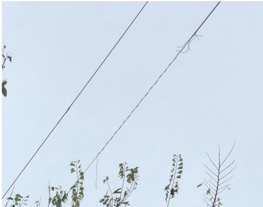
Damaged or Frayed Conductor
